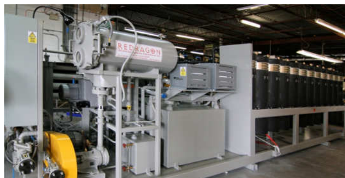
Above: TORS-4000, skid-mounted
